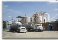
Bulk Gas Storage
