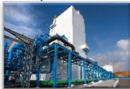
Air Separation Unit
